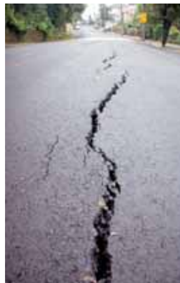
Rachadura enorme na Rua João Werlang
